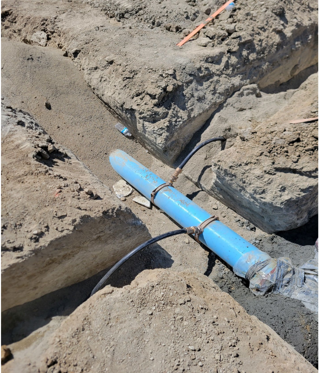
( New water main lines being installed at the housing tract off of Orange st / 35 th st , north of Howard st)
