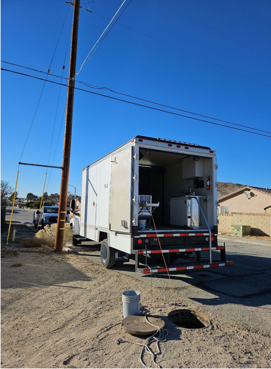
Sewer Camera truck in action
