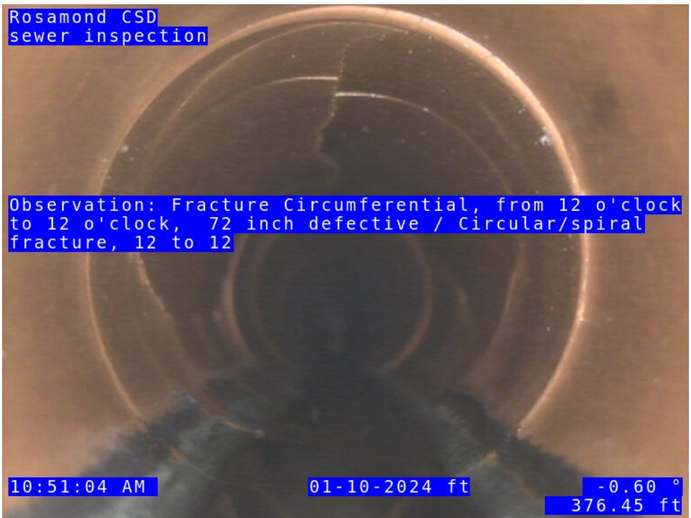
Camera footage from C and B street sewer main.
