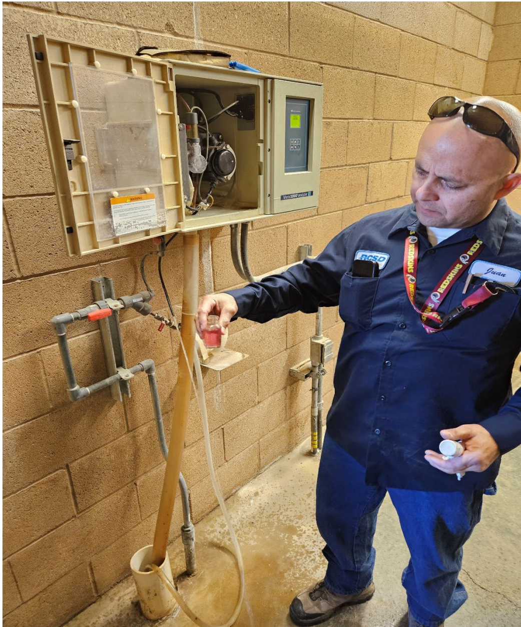
Operator Juan De La Rosa checking system cl2 residual for public safety
