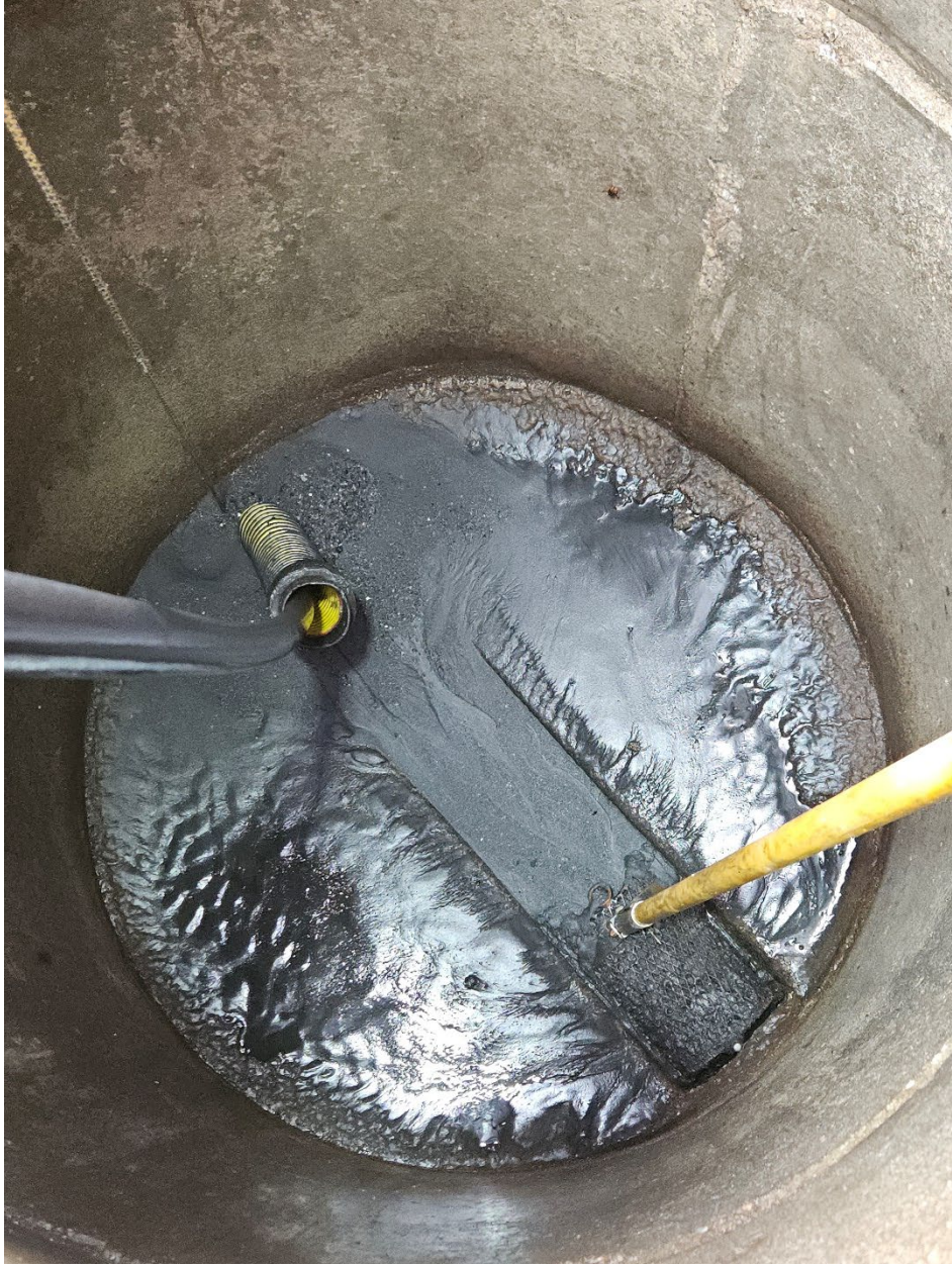
Grit that was pulled out of our sewer system on phlox ave
