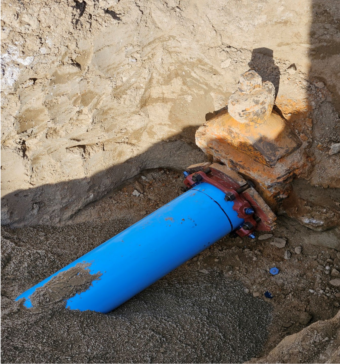
New pipeline being tied into our system on Christy ave at the Legacy development
