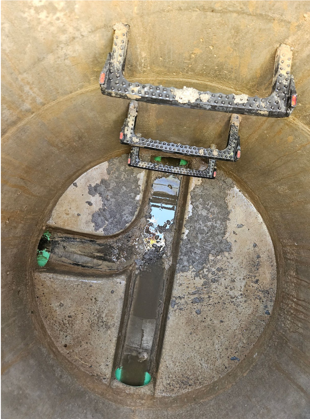
Concrete left in manhole by contractor causing flow issues
