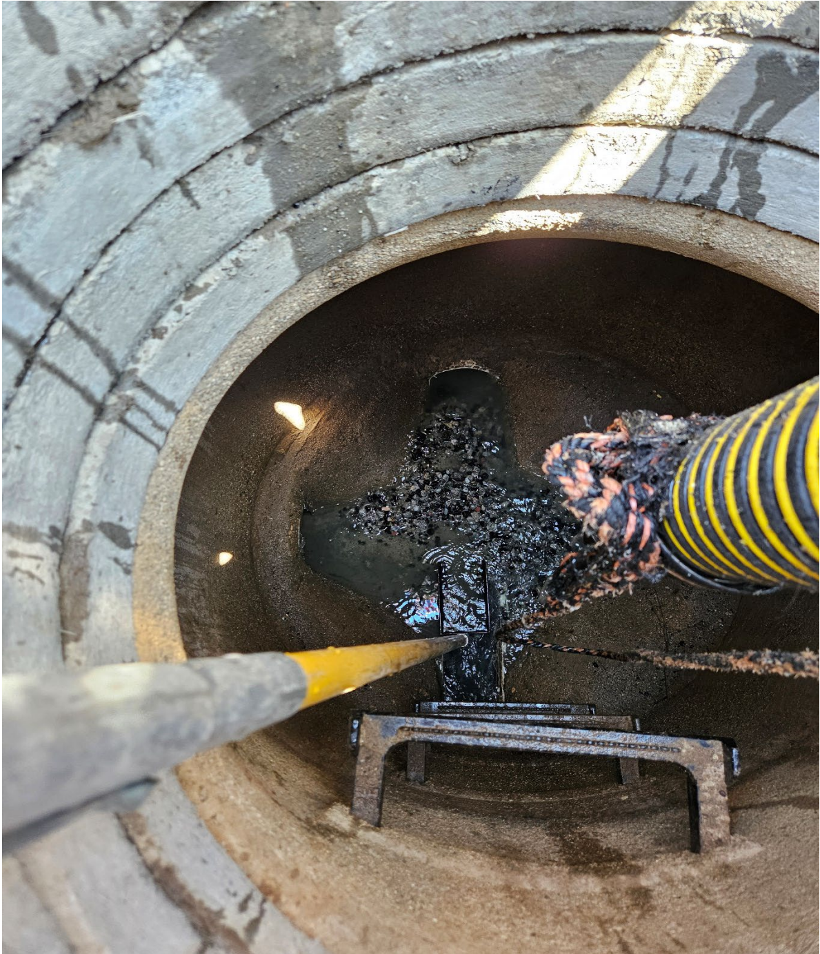
Debris found in our collection system being removed
