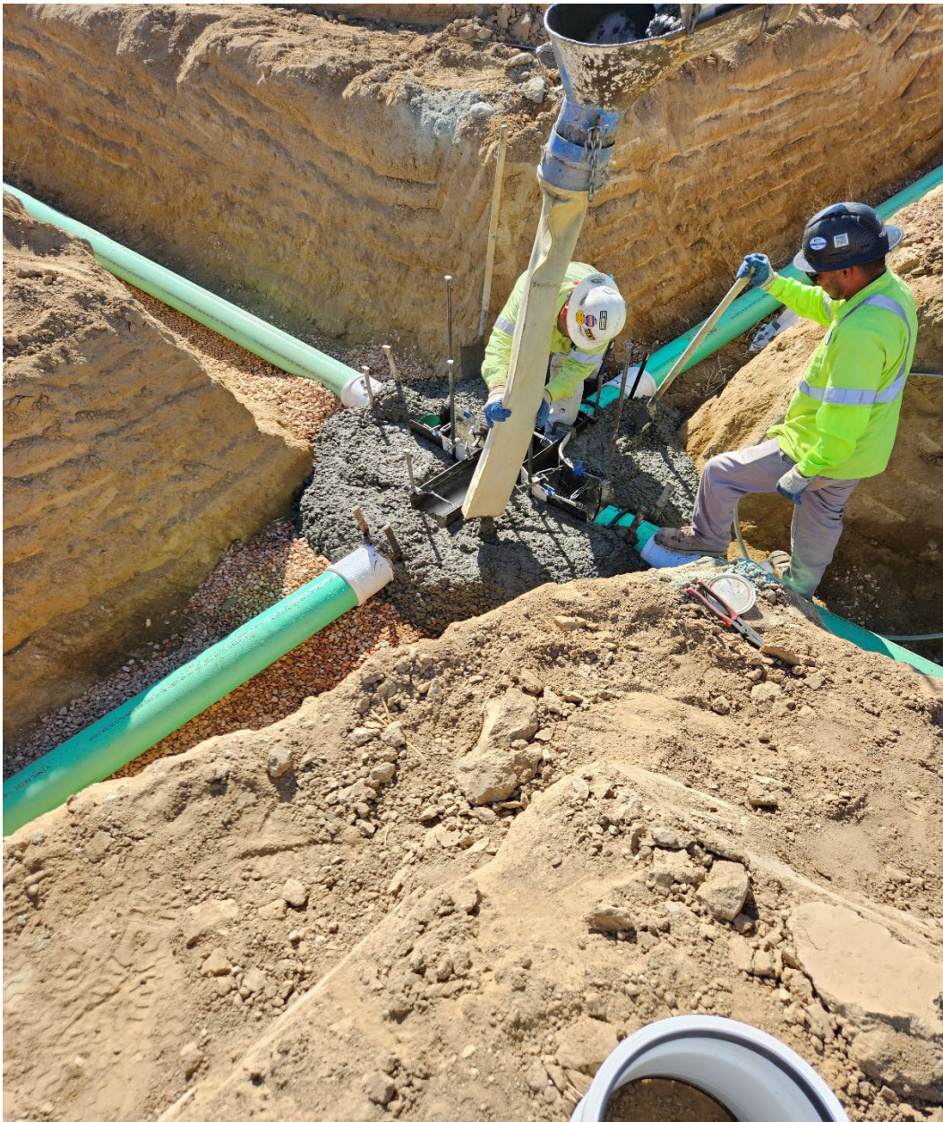
New sewer manholes being poured by Tejon construction for the new Hillview Homes development off of Stetson Ave.
