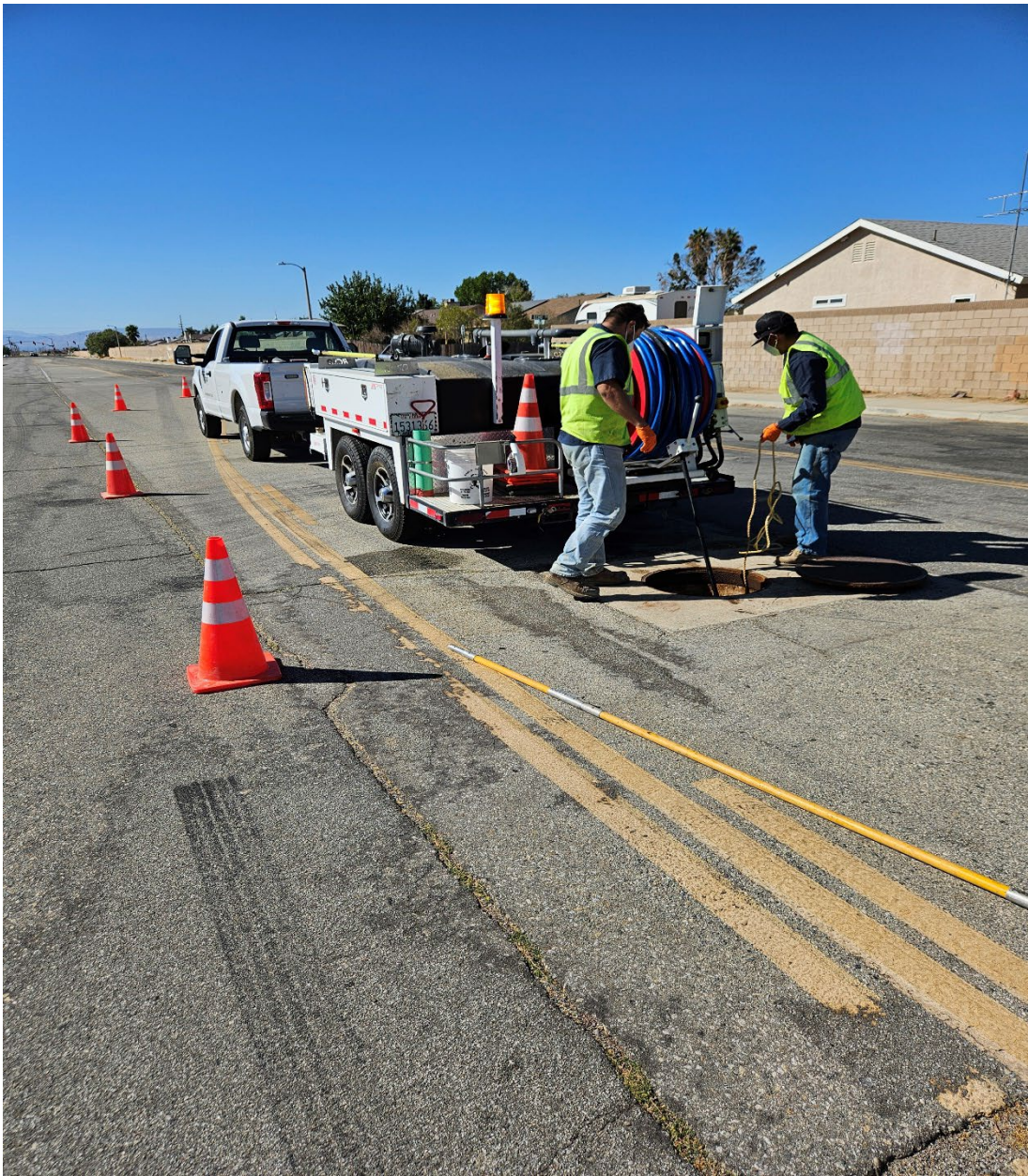
Public works staff cleaning the sewers on one of our trunk lines on 30 th st west.
