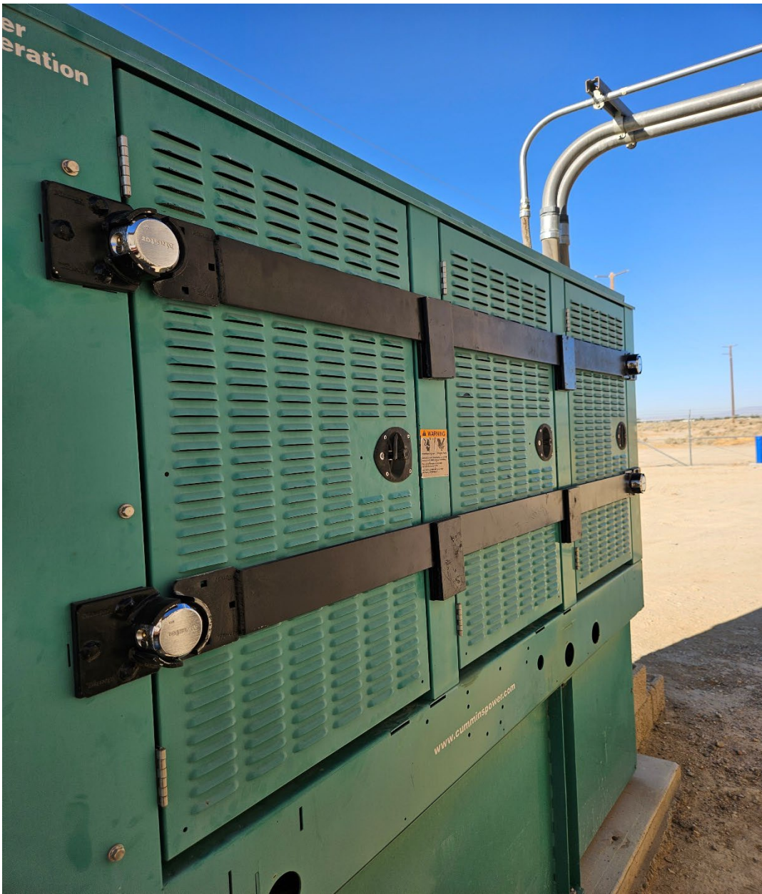
Anti-theft locks and cages fabricated by the public works dept to prevent break ins and fuel theft on our generators.
