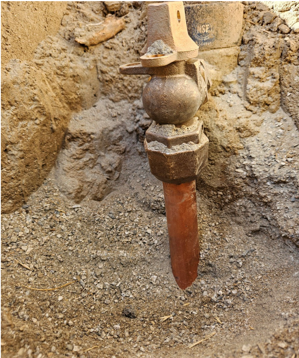
Brand new copper service lines and angle stop shut off valves installed by Lyles construction on the Trakell tract.
