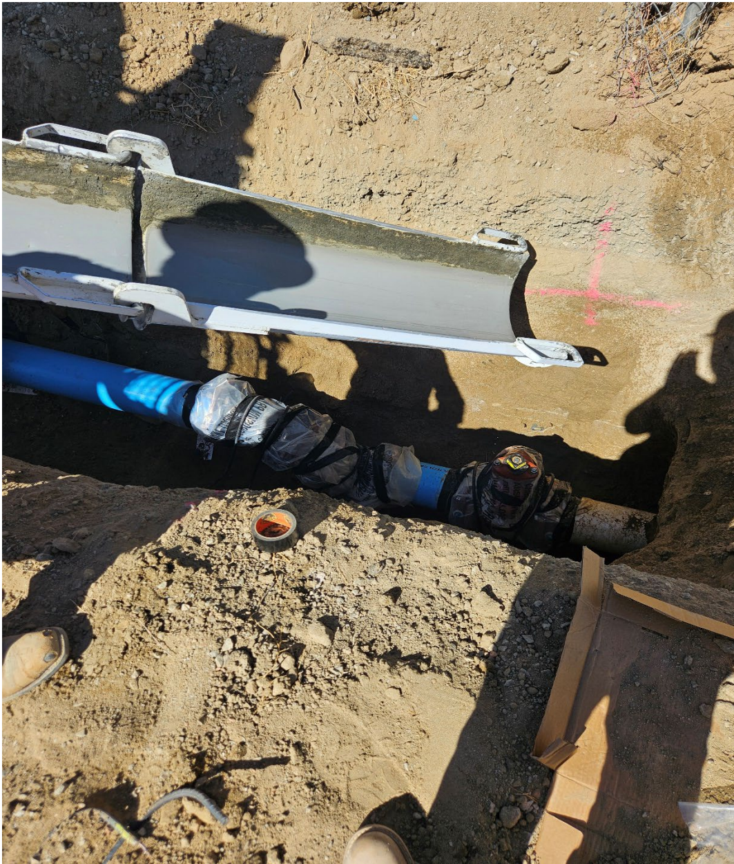
Water main line tie-in by BCI Construction for the new K.Hovanian development at the West side of the 3000 block of Poplar ave. The white pipe is existing and the blue pipe is new. They are pouring a concrete thrust block around the new valve.
