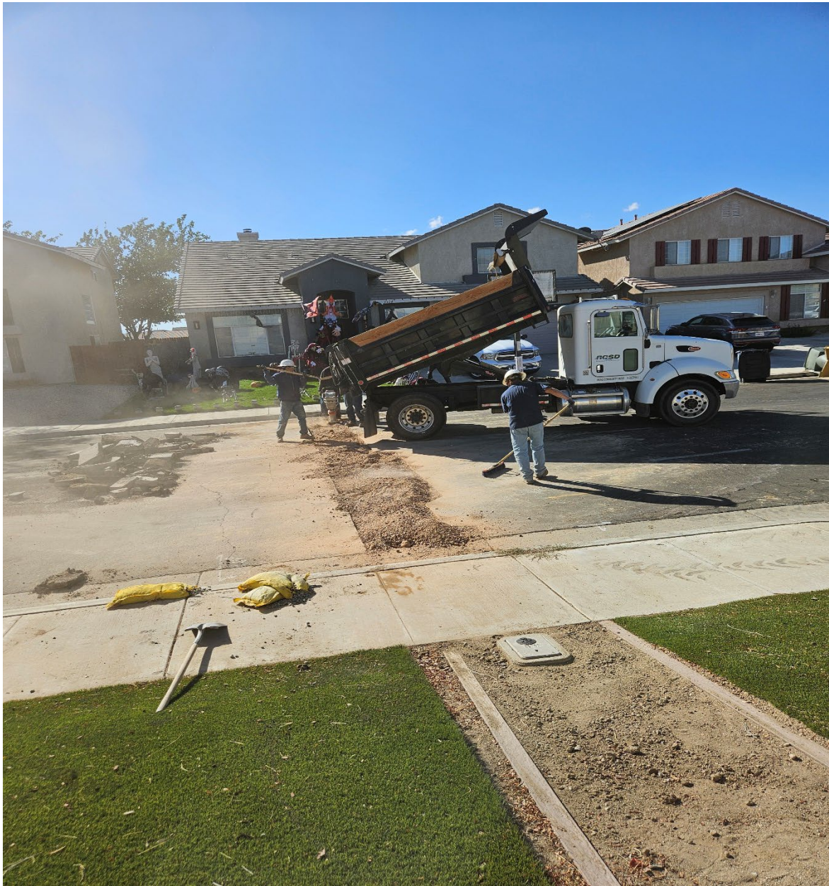
Public Works dept replacing service lines on garnet ave. We have been focusing on installing new lines at problem locations on this street.
