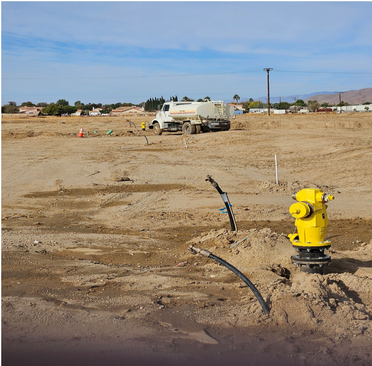
New water infrastructure installed by Tejon Construction for the next tract development by Hillview Homes.
